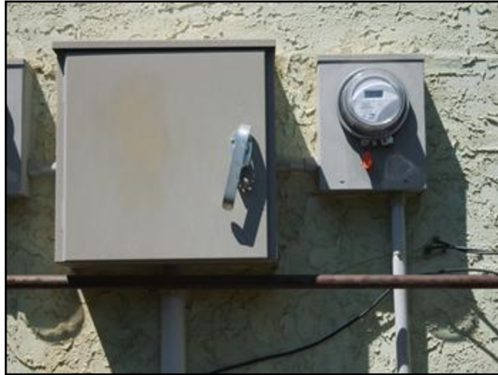
17. Main power coming to the house
