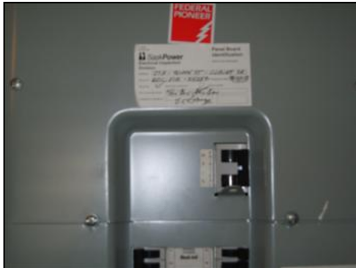
18. Main disconnect in basement
